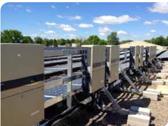
> 1MW, Ontario, Canada
