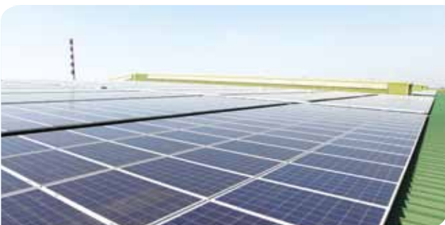
> 50MW Baosteel, Shanghai PV rooftop power system
