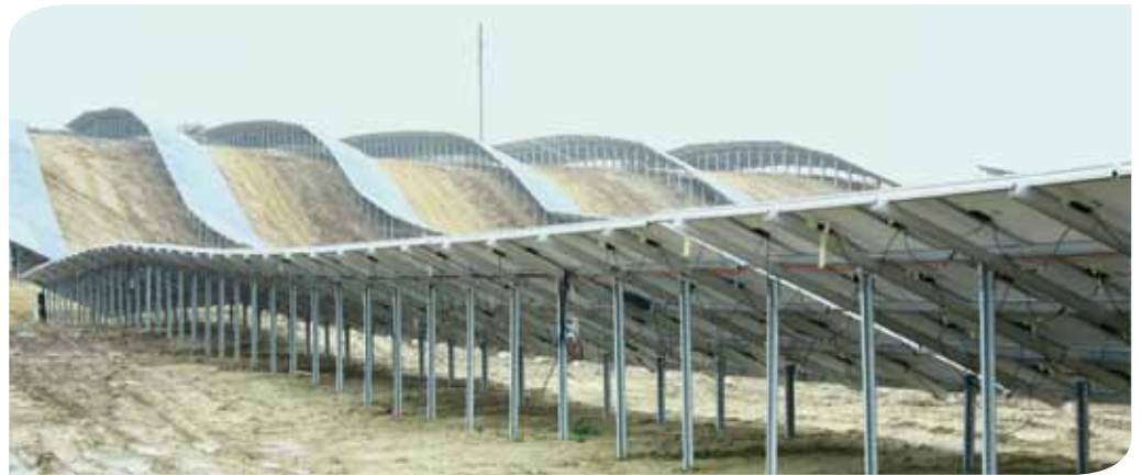
> 2.4MW, Friedland & Neuheilenbach, Germany
