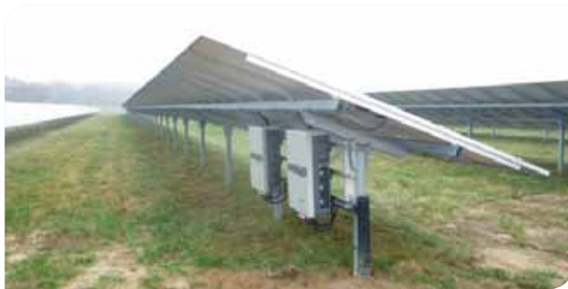
> 10MW, Domsühl, Germany
